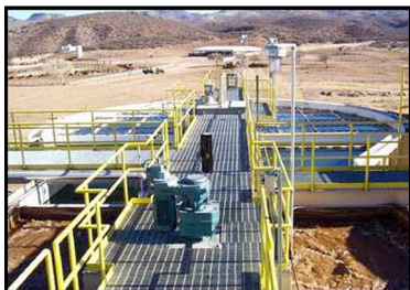
Overview of Water Treatment Plant at Lower Pinal Creek.
